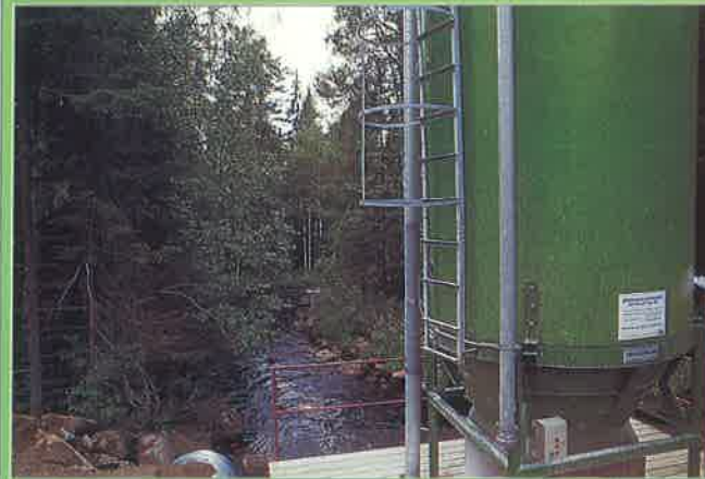
Above: Lime towers in Sweden dispense lime to help neutralize acidic water in lakes.
