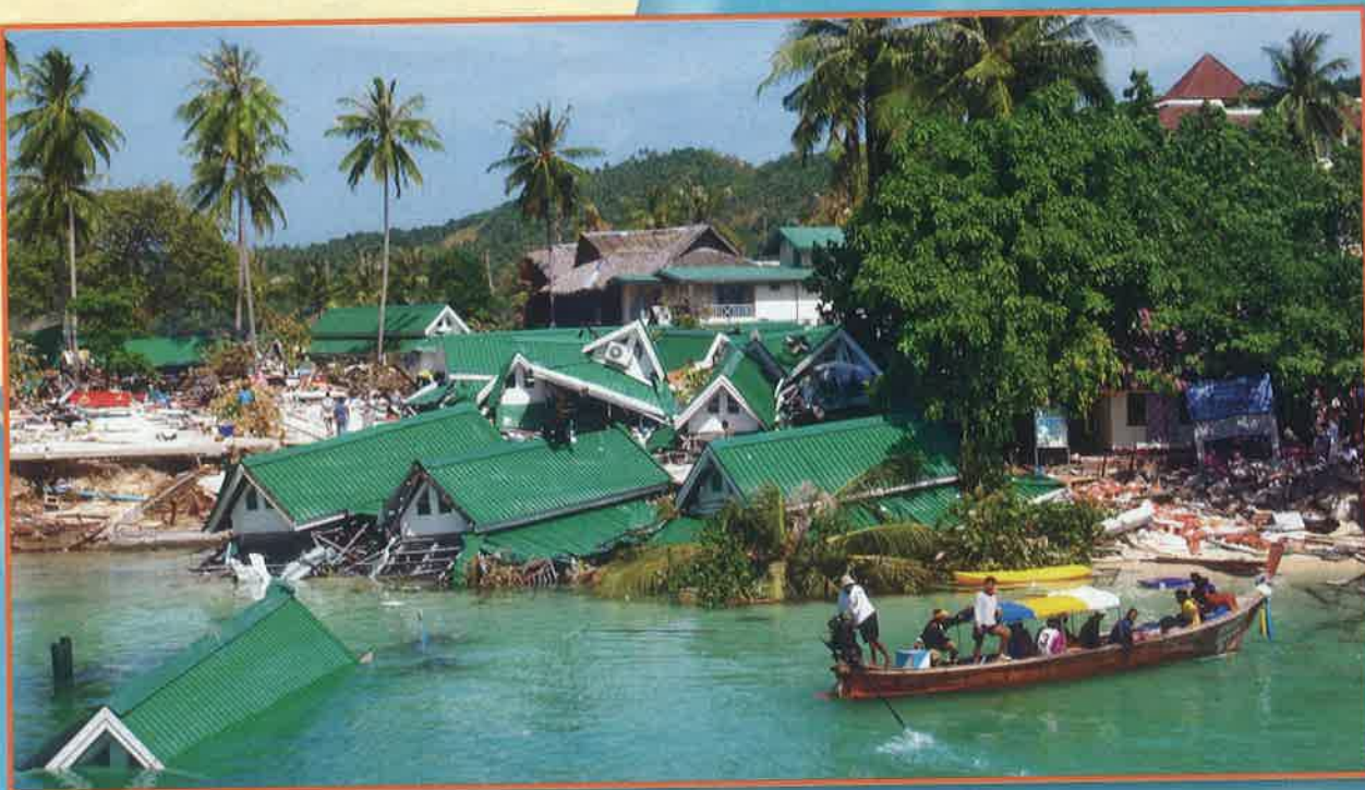
Wrecked by Water. In December 2004, a powerful tsunami destroyed this hotel in Thailand.
